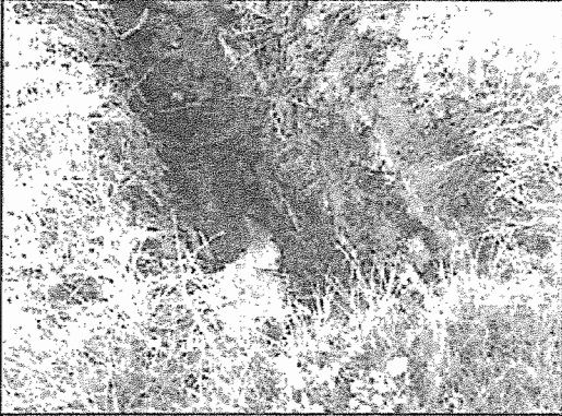
Photo #9 Test Pit 3 measured 13 feet in length, 4 feet in width, and was 15 feet deep. Water was observed in the test pit. Significant rainfall occurred prior to and during the excavations.
