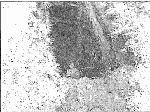
Photo #3 Test Pit 1 measured 14 feet in length, 4 feet in width, and was 15 feet deep. Water was observed in the test pit. Significant rainfall occurred prior to and during the excavations.
