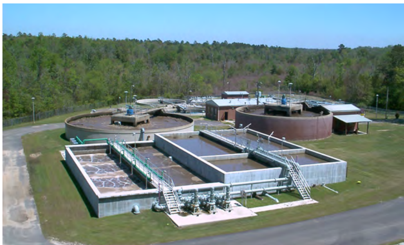
Quincy Wastewater Treatment Plant.
