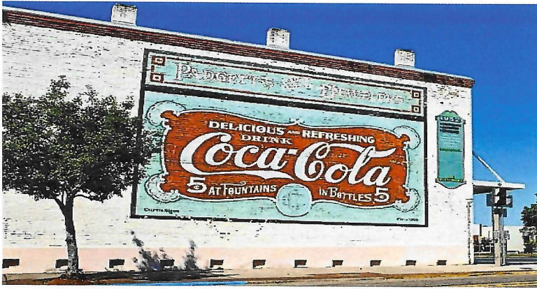
Figure 2. shows the current conditions of the mural and the surrounding streetscape. Currently, the mural is fading, chipping, and in need of touch-up work. Mural Size Dimensions: 31 feet wide and 21 feet high, square footage: 651 feet.
